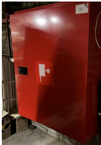
Fire hose reel in hose cabinet
