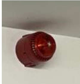
Alarm siren with flashing light
