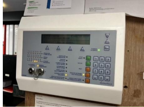
Fire detection control panel
