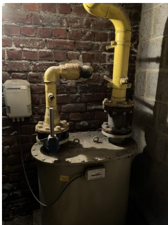
Main gas shut-off valve
