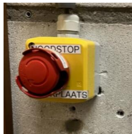
Emergency shut-off valve – boiler room
