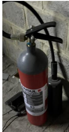
CO 2 fire extinguisher
