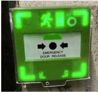
Door release (Technical room above the theater hall)
