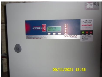
Gas detection panel
