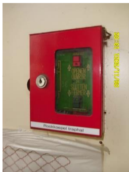
Smoke vent control
