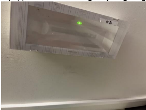
Autonomous emergency lighting fixtures (activate in case of power failure)
