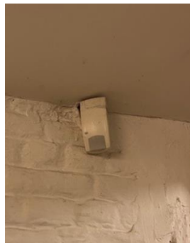
Alarm system sensor
