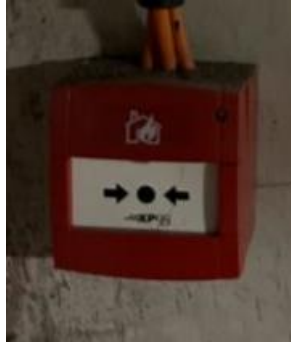
Manual fire alarm button
